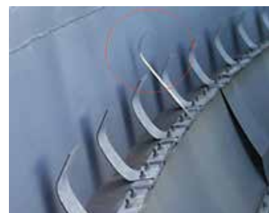
Typical shunt which has lost contact with tank shell
