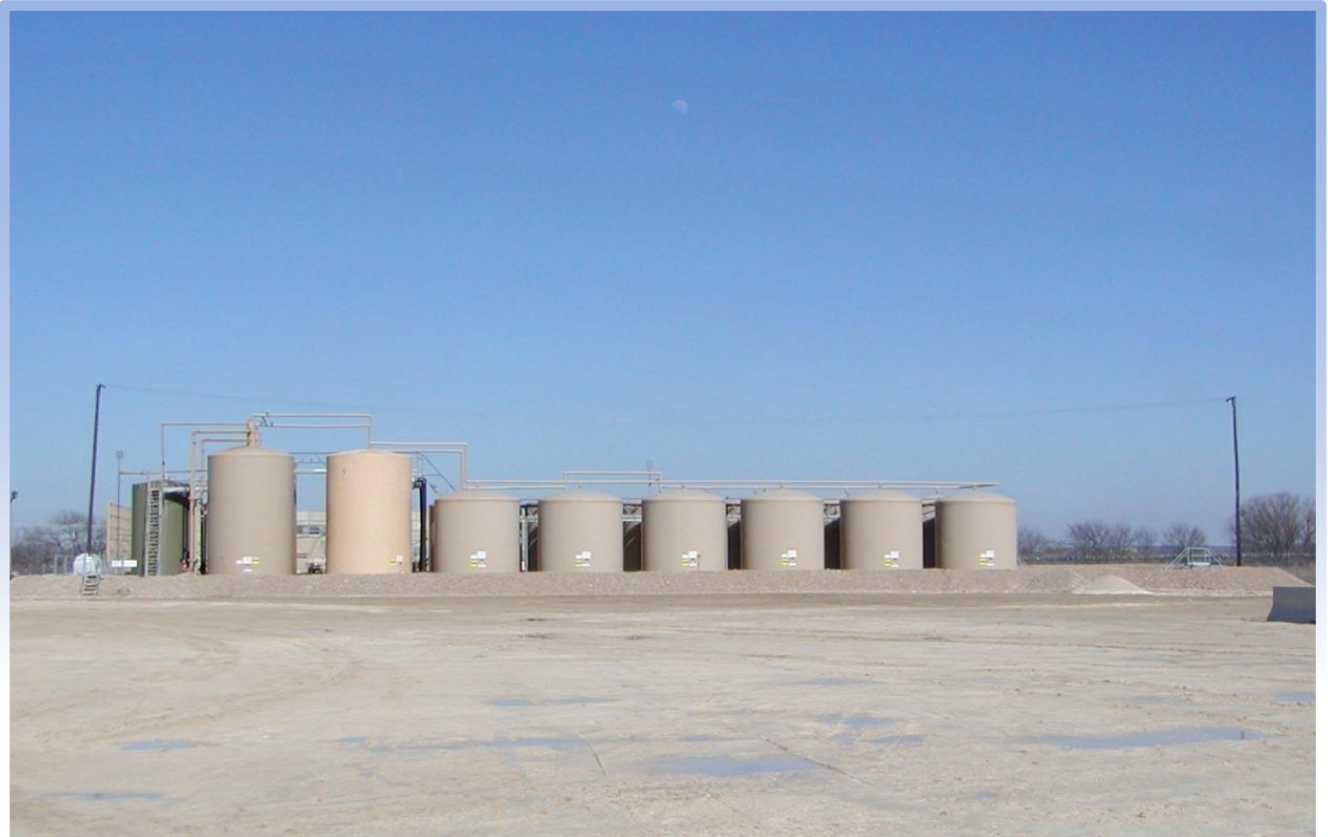
Typical SWD site with oil, gunbarrel, sand and salt water tanks
