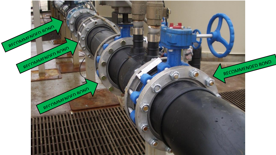
Isolated metallic objects within containment wall
