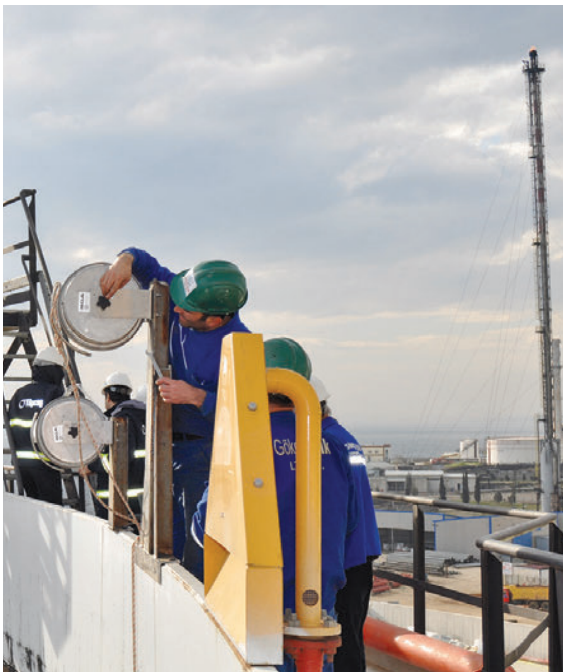
Workers install one of patented dissipation array system systems designed, engineered and built by Lightning Eliminators and Consultants Inc. - Photo Submitted
