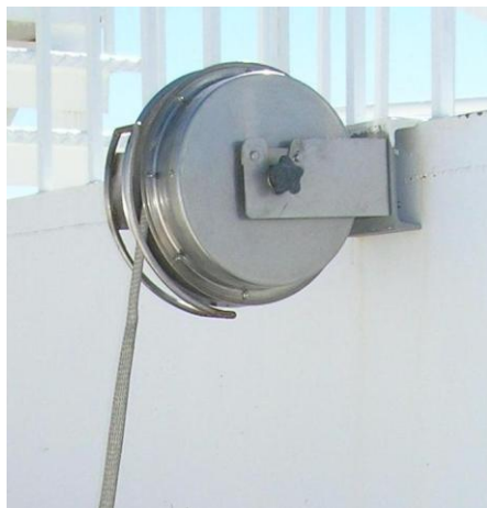
Figure 4: LEC Retractable Grounding Assembly (RGA) on Floating Roof Tank
