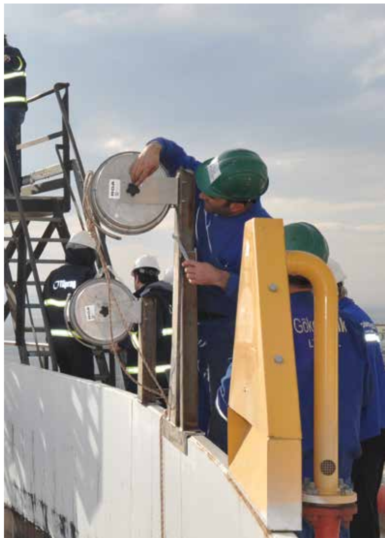
RGA installation on floating roof tank
