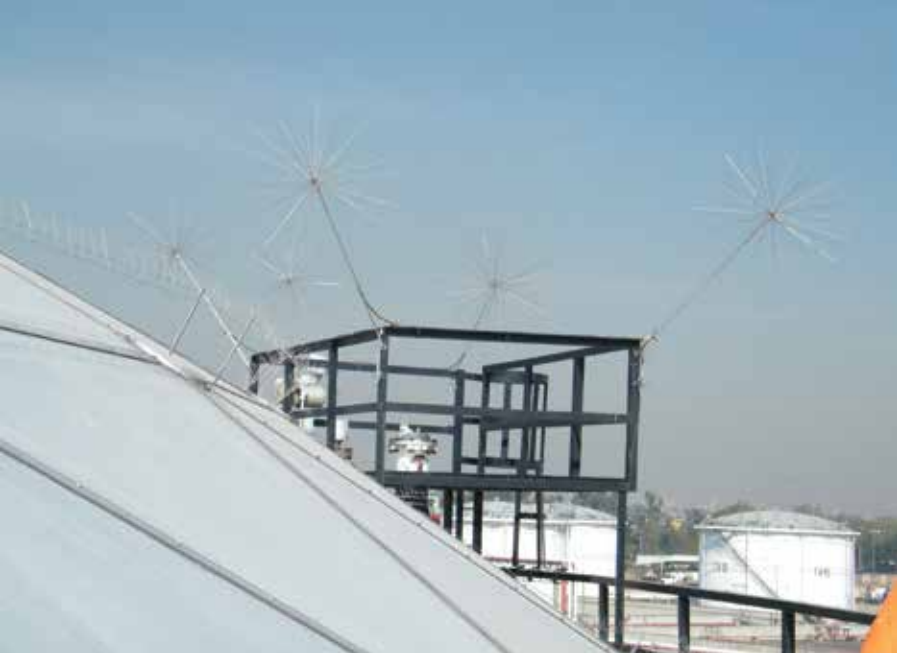
DAS lightning protection with spline ball ionizers protecting a tank farm
