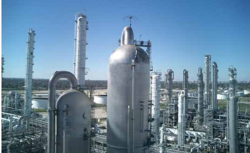
Dissipation Array System (DAS) protecting BASF
