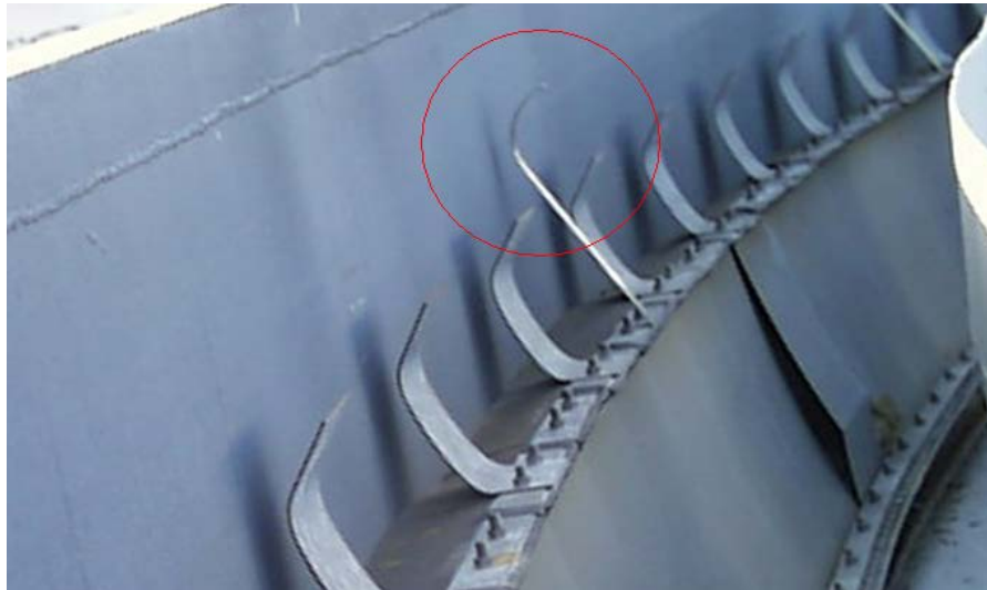
Figure 6: Shunt Not Making Contact with Out-of-Round Tank Shell
