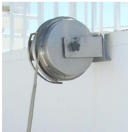
Figure 9: LEC Retractable Grounding Assembly (RGA) on Floating Roof Tank
