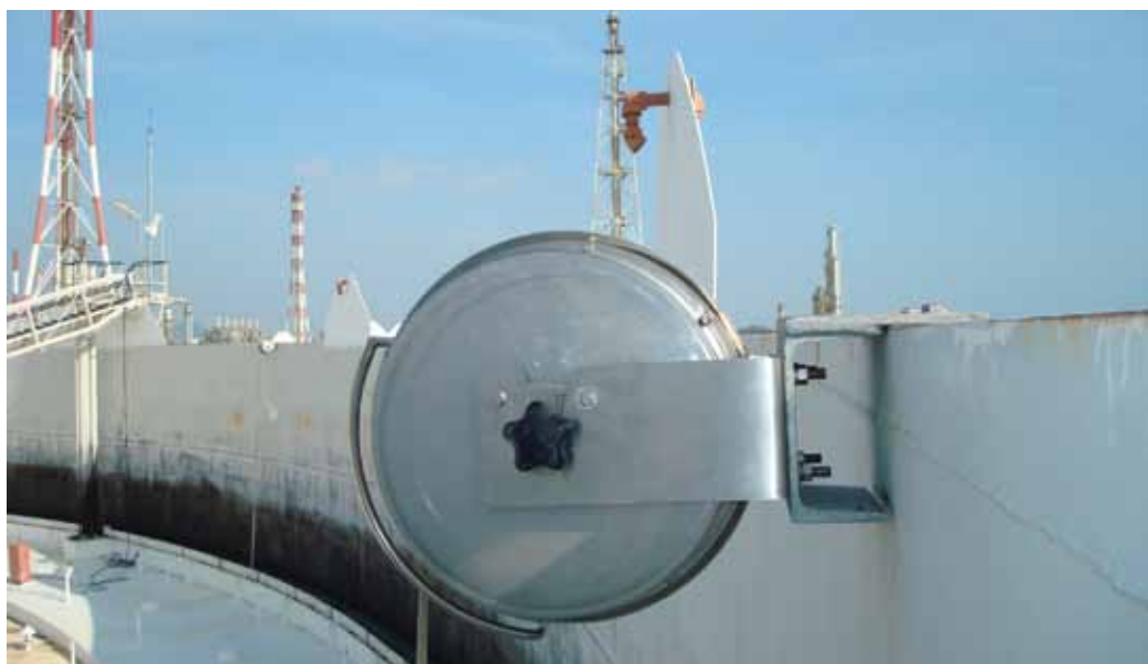
A RGA on a floating roof tank
