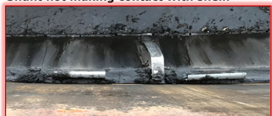
Sludge on shunt and rust on inner shell wall.
