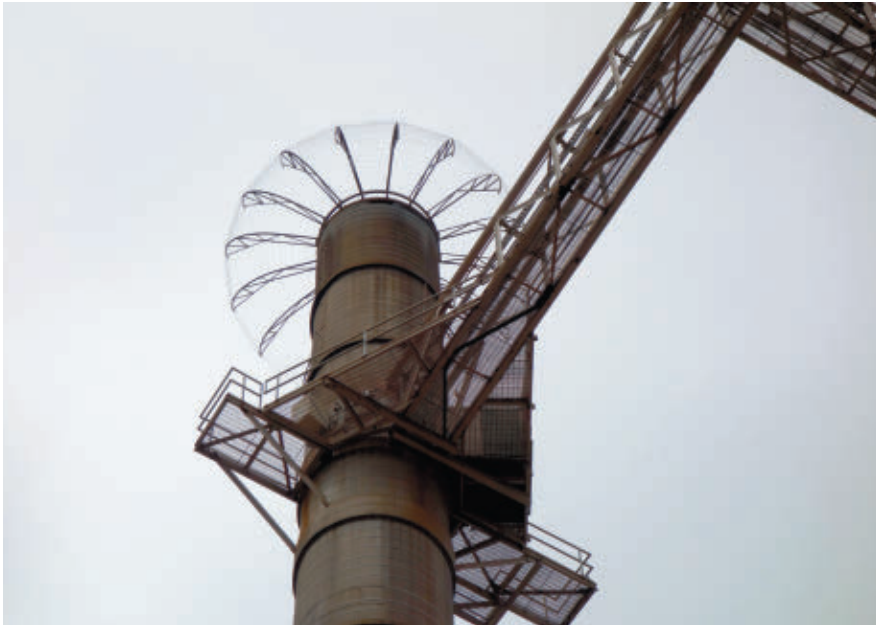
Protective systems—such as lightning avoidance, grounding networks, and surge protection devices—are considered essential in pulp and paper mill design.
